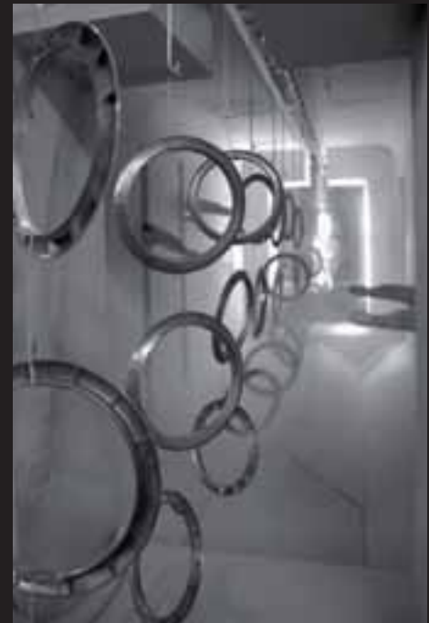
Automatic installation of tunnel for defosfating and degreasing, powder coating booth and polymerization oven.
