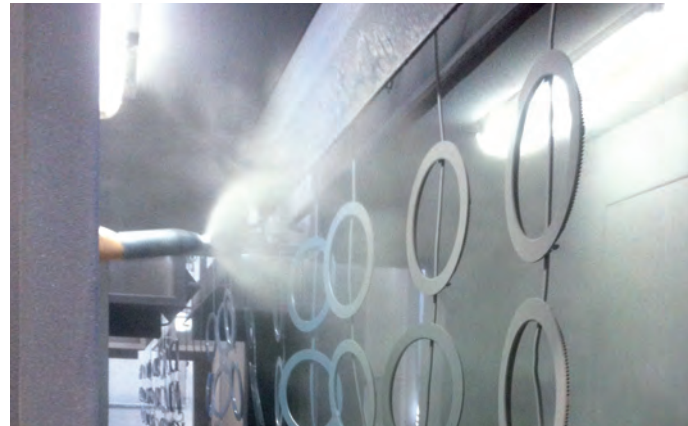
Automatic installation of tunnel for defosfating and degreasing, powder coating booth and polymerization oven.
